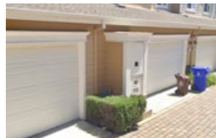
Wherever possible, mechanical/utilities equipment should be placed in alleys. In this example, they are further shielded by architectural elements and a hedge.
