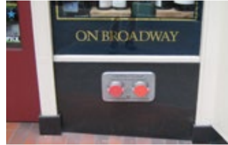
Example of an appropriately placed double standpipe connection in the base of a building at the sidewalk.
