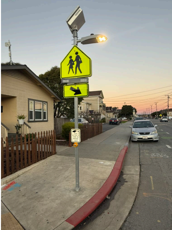
Rodriguez St & Kearney St RRFB at Radcliff School Installed January 2025 $15,000
